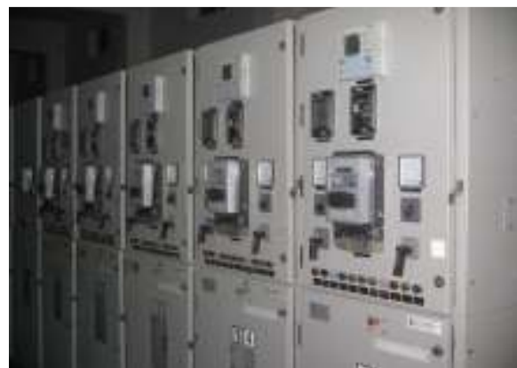
ET Substation - ready to be charged
