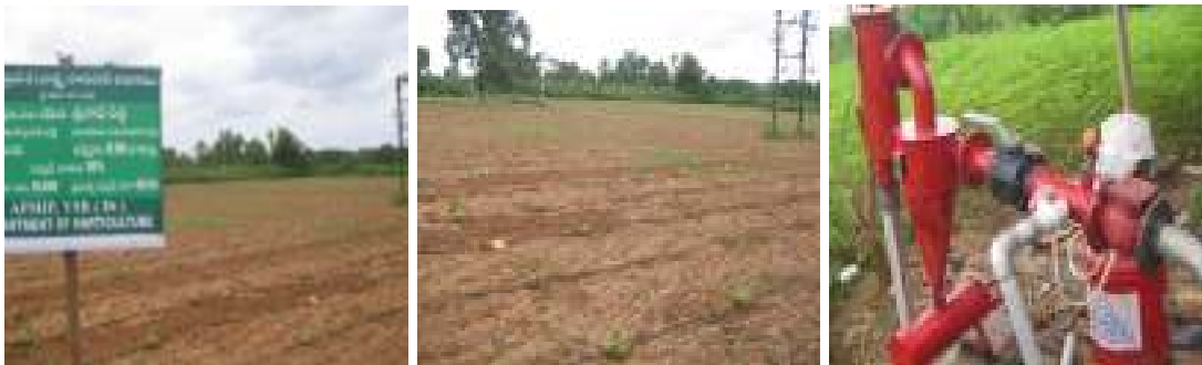
Drip irrigation system for banana
